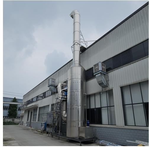
碱喷淋塔+三号车间排气筒
